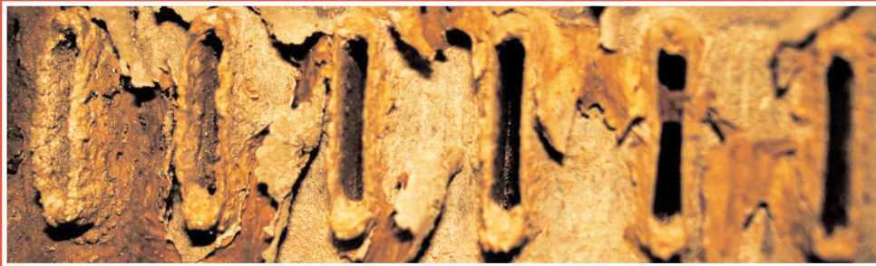
Harmful mineral scale and oxide deposits
